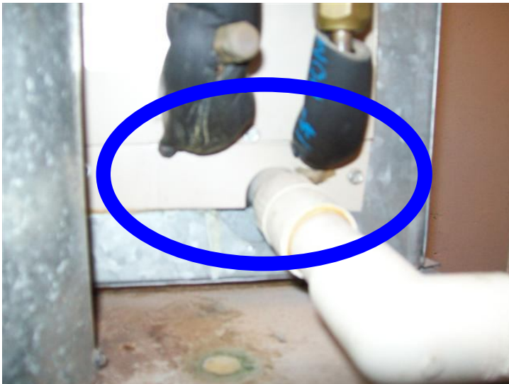
Equipment: HVAC System
