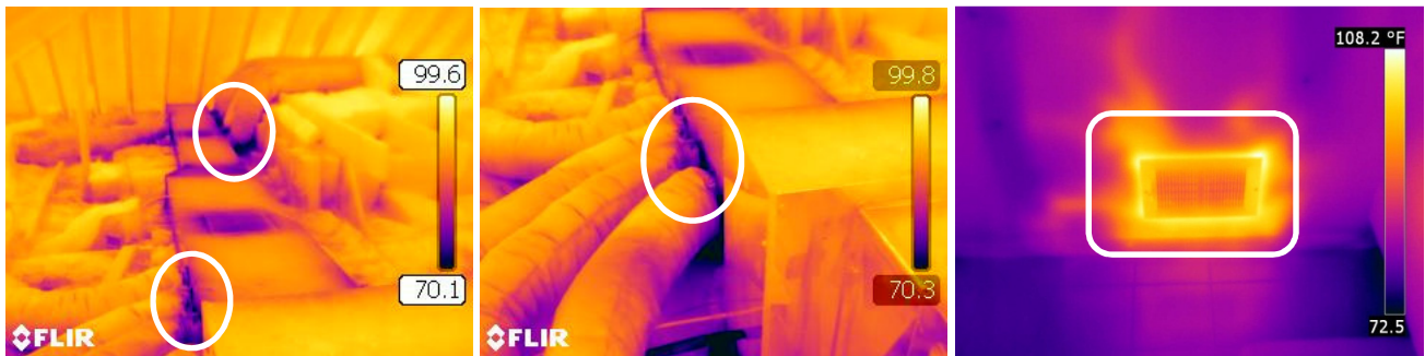
Leaking duct connections
