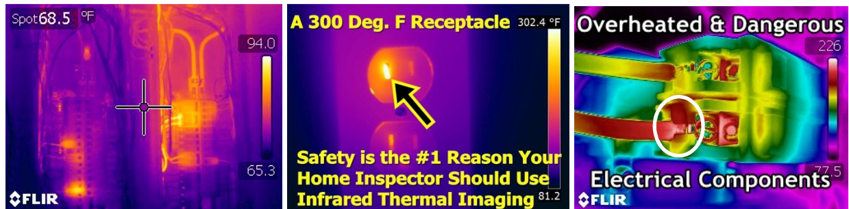
Dangerous electrical conditions
